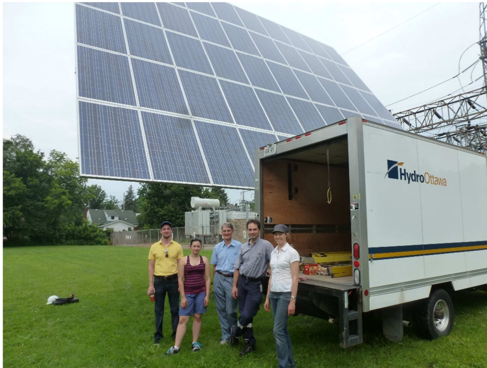
Pictures from three Hydro Ottawa photovoltaic installations: preceding page - view of Merivale Roof 20 kW array; above - Bank St. pole-mounted 1.56kW system, with Sara Benedet (Sunlab) on ladder taking shadow measurements, Al Lemay (Hydro Ottawa) assisting, and Sasha McCollough (Energy Ottawa) in background; bottom – Riverdale 2 axis tracker 10kW, with Allan Morton (Energy Ottawa), Sara Benedet, David Wright (uOttawa), Al Lemay, and Joan Haysom (uOttawa).
